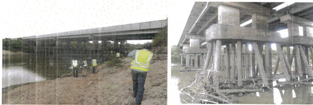
Plate. 1.2 Scouring of Bridge Foundations
