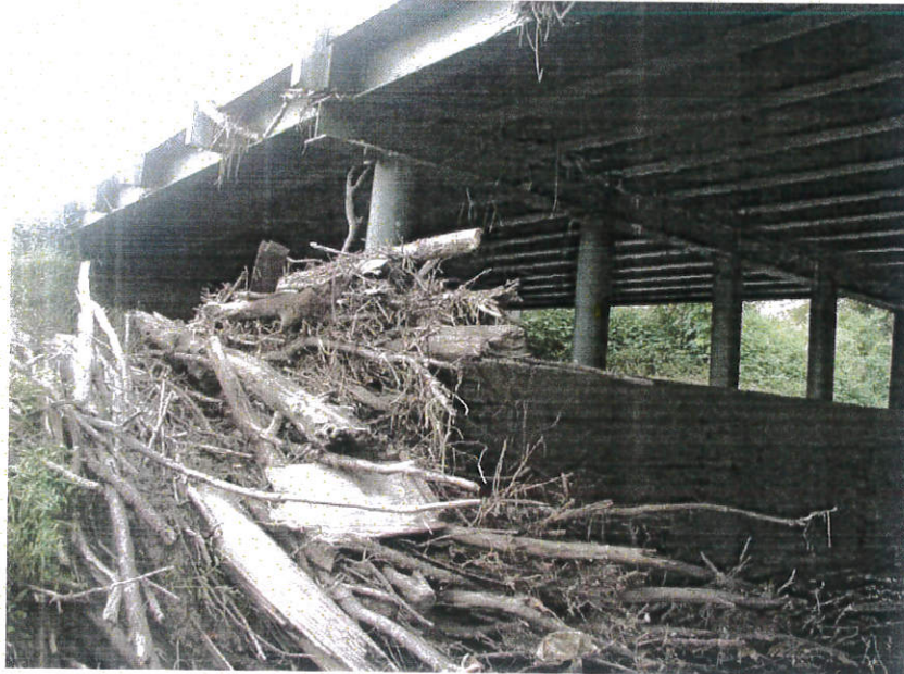
Plate 2.23 Woody debris at a bridge pier. Note how debris can be much wider than the pier itself (also note debris on lower chord of bridge deck). Source: NCHRP Web-Only Document 48 (see NCHRP 2010a).
