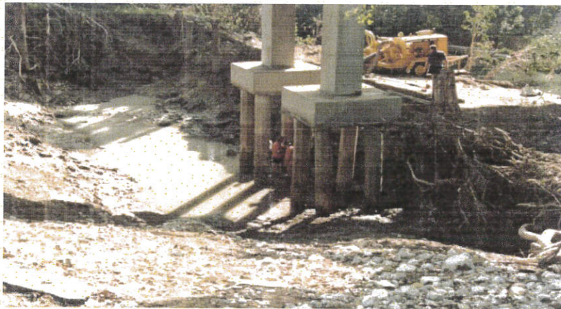
Plate 1.1: Local scour damage at piles on the Logan River
