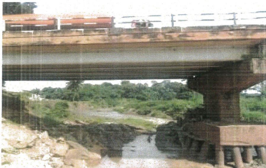
Plate 1.5; Ekulu River Bridge in Nigeria; pier foundation threatened by scour.
