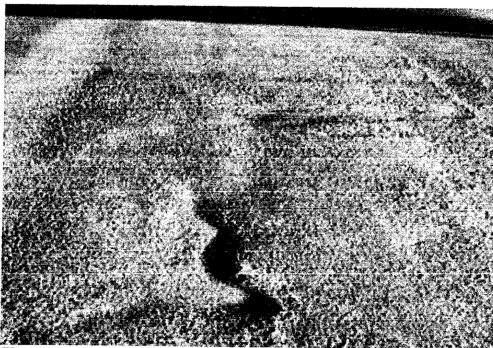
Plate 2.2 Shoving on a trafficked road, (Smith, 2004)
