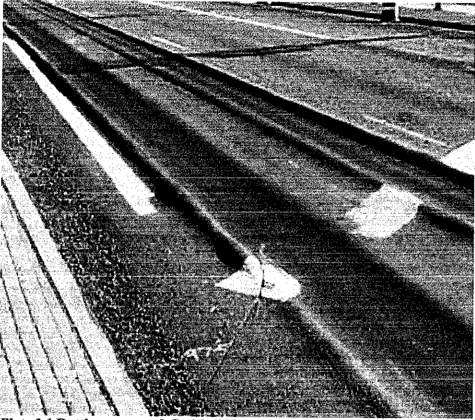
Plate 2.1 Rutting on a road, Smith (2004)
