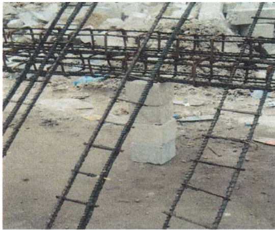
Figure 3: The arrangement of bamboo in the foamed aerated concrete beam without shear links
