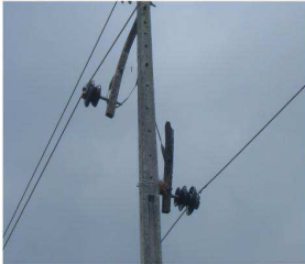
FIG 3. 11Kv line with a Slanting cross arm.
