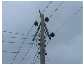
Fig 4. 11kV Line with a cross arm.
