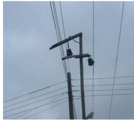
Fig 2. Wooden Pole with a Broken Wooden Cross-Arm.
